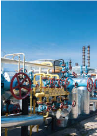
The company's gas detection and monitoring technologies help to enhance safety in the oil and gas sector.
