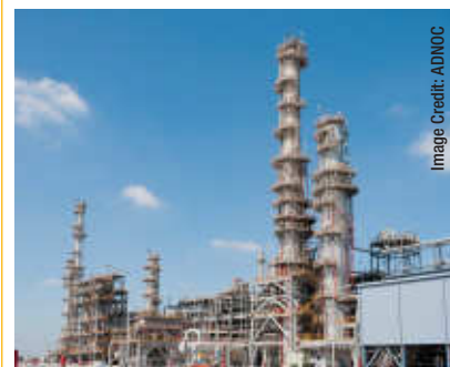
ADNOC is also driving industrial growth with the expansion of its downstream business.
