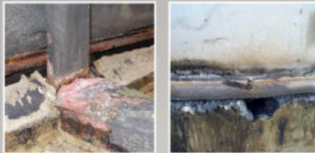
COMMON CORROSION PROBLEMS
