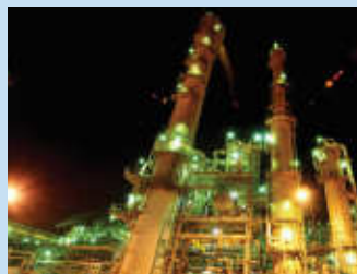
The facility will meet growing domestic and international demand for this clean and versatile chemical commodity which is gaining momentum as a lower-emission fuel alongside existing uses spanning industrial products.
